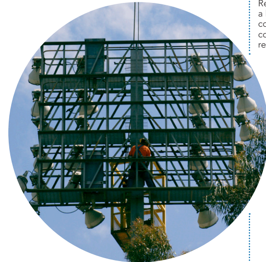
Stadium Lighting California Electrical Contractors' Association Design Award
